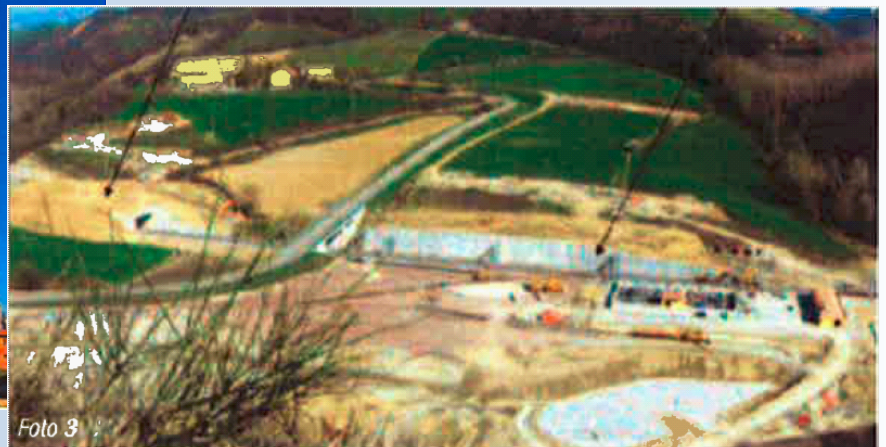
High speed railway between Bologna and Florence: landslide Laurenziano
